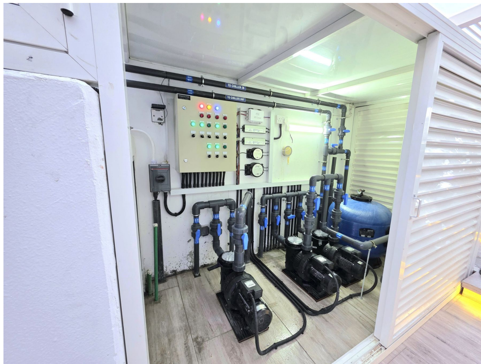
PUMP ROOM • PUMPS, FILTER & CONTROL PANEL
